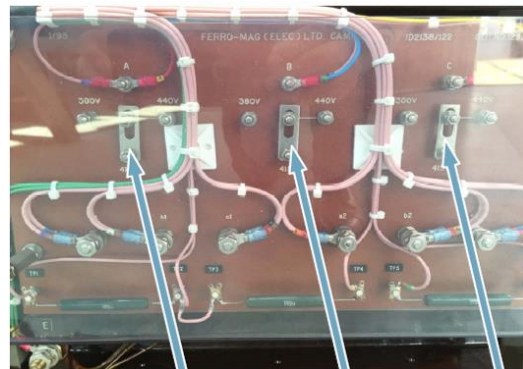
VOLTAGE (440 V/415 V/380 V) SELECTED BY SETTING THREE LINKS ON THE TRANSFORMER AT INSTALLATION.
